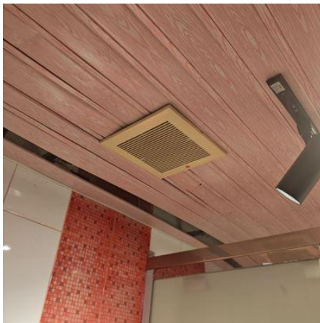
Bathroom - Exhaust Fan 10/05/2025 18:27
