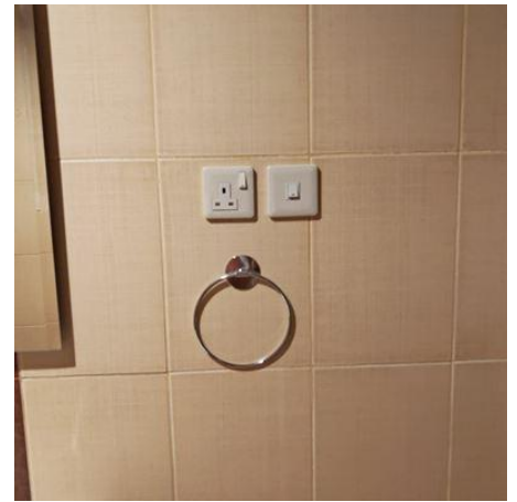
Bathroom 2 - Power Points 10/05/2025 18:41
