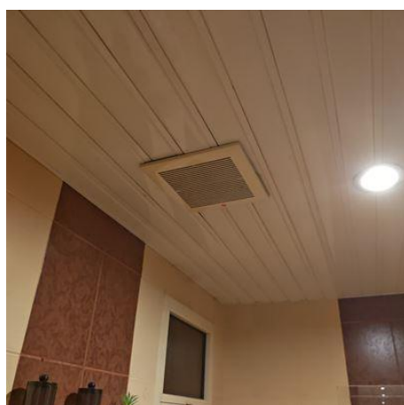
Bathroom 2 - Exhaust Fan 10/05/2025 18:39
