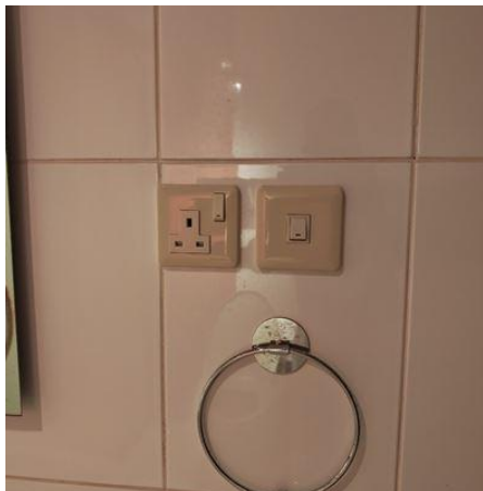
Bathroom - Power Points 10/05/2025 18:32
