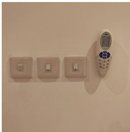
Bedroom 2 - Air conditioner 10/05/2025 19:20
