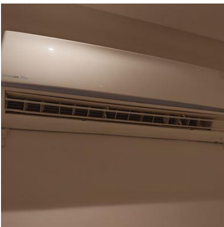
Bedroom 2 - Air conditioner 10/05/2025 19:20
